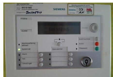
Alarm panel on the 1st floor
