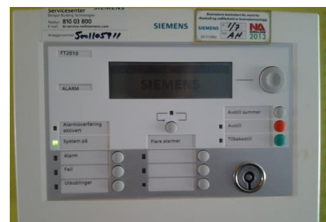
Alarm panel on the 1st floor
